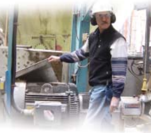
In paper factories, motors are treated mercilessly: mechanical damage, contact with aggressive chemicals and around the clock operation are the norm.
